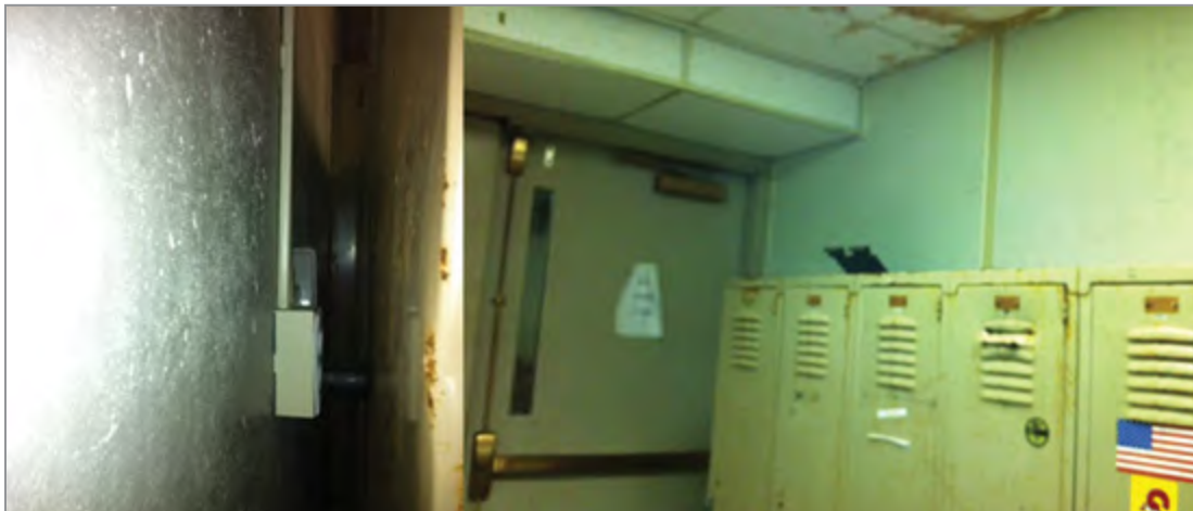
Figure 4. HomeFree Door Alarm System Blocked Off and Rendered Non-functional at AFRH-W Source: DoD IG–SPO
